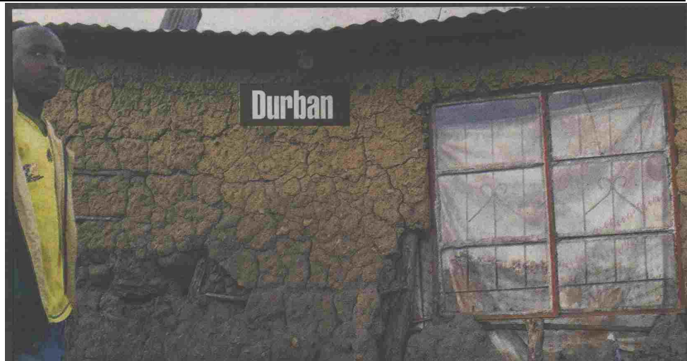
Nhlanhla Shange stands outside his damaged house.
